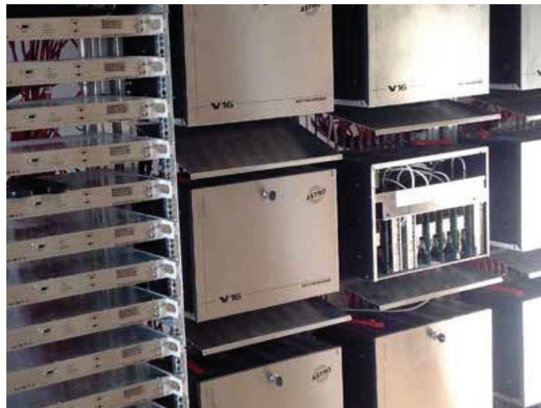
A look at our in cable headend in Wilhelmshaven
