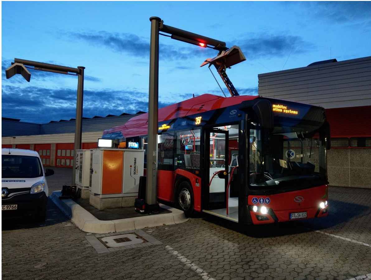
Charging Station Freiburger Verkehrs-AG
