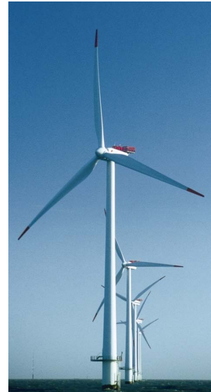
Offshore wind farm
