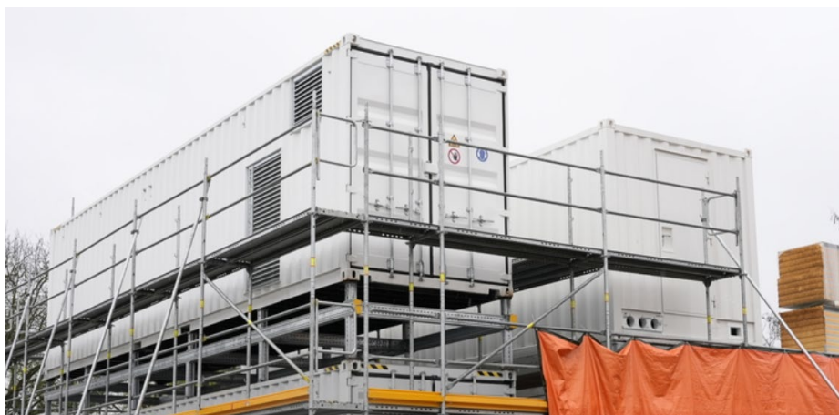
Figure 4: Electrical Control Centre successfully installed in April, enabling commencement of Electrical Workfront.
