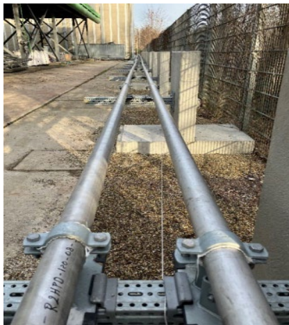
Figure 2: Brine line installation and construction progress at Vulcan's Lithium Extraction Demonstration Plant at Landau.
